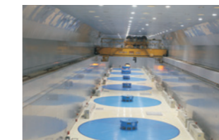
The underground power plant of Three Gorges began power generation.
