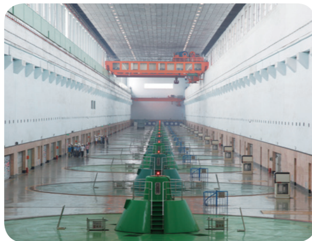
Gezhouba Hydropower Plant
