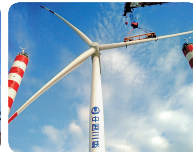
The turbines of the Xiangshui Offshore Wind Power Project were hoisted and installed.
