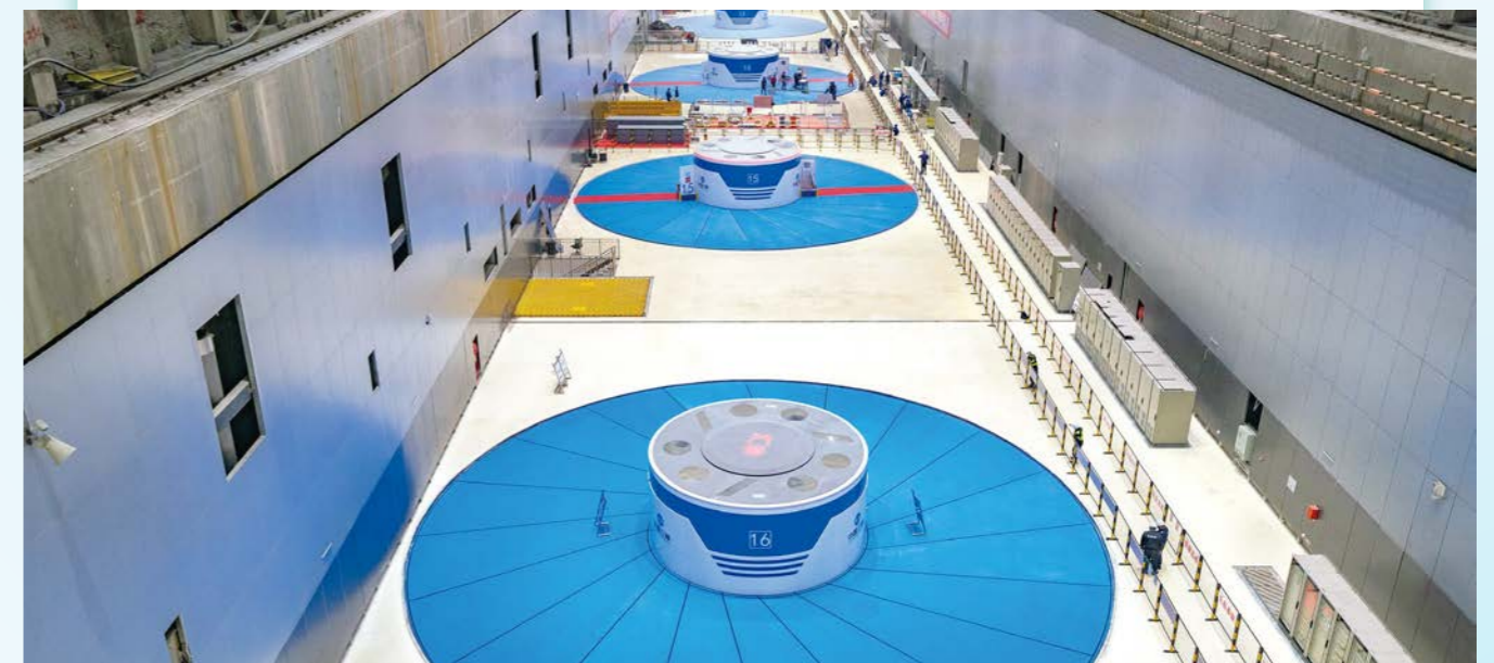
Main plant of the underground power station on the right bank of the Baihetan Hydropower Station
