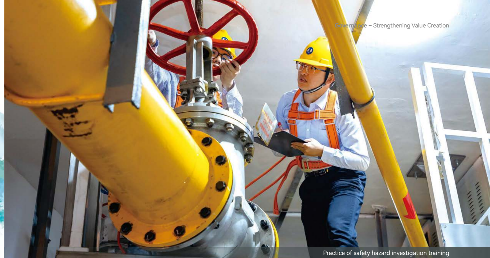
Practice of safety hazard investigation training
