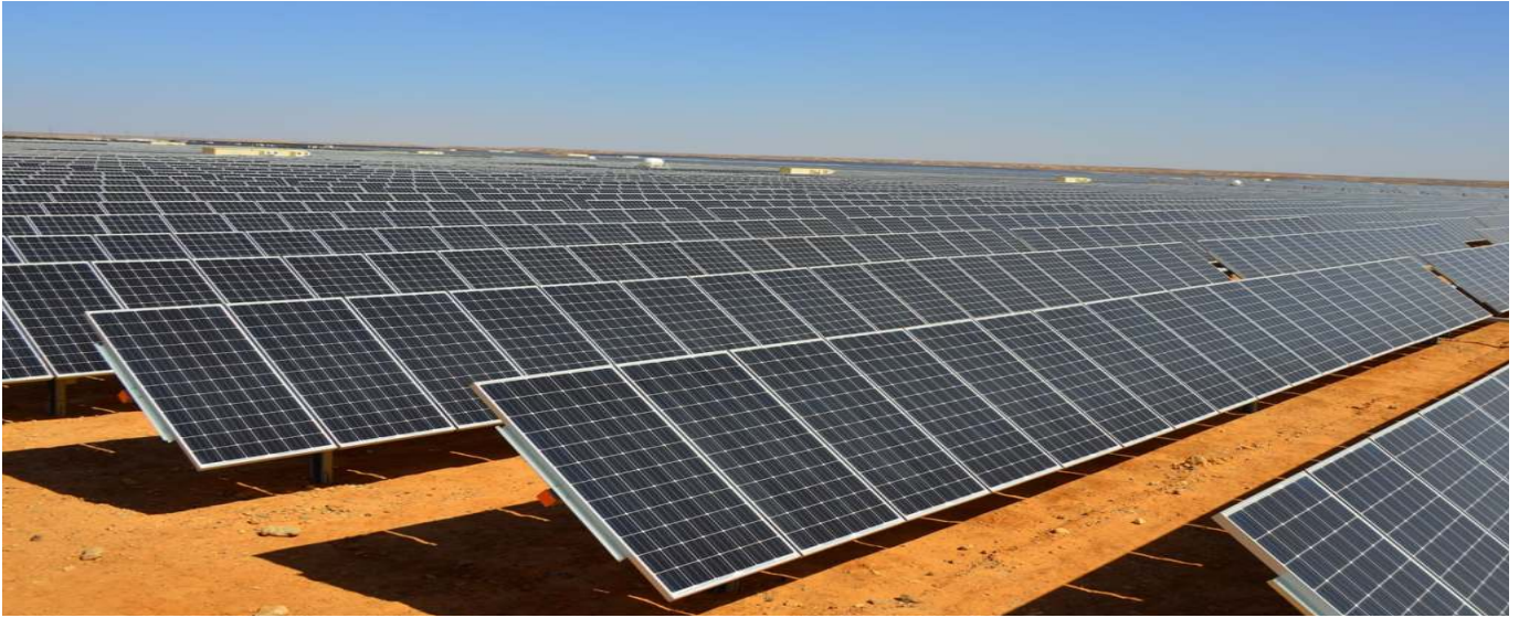
Panoramic View of Ma'an Solar PV Project
